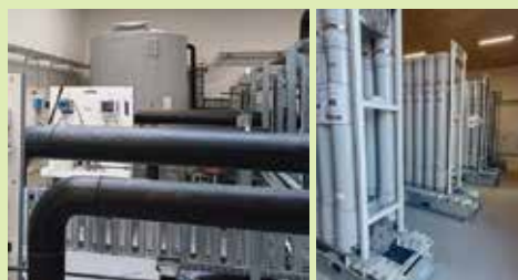
Warm Water Tank for Cleaning Membranes with some instrumentation.
